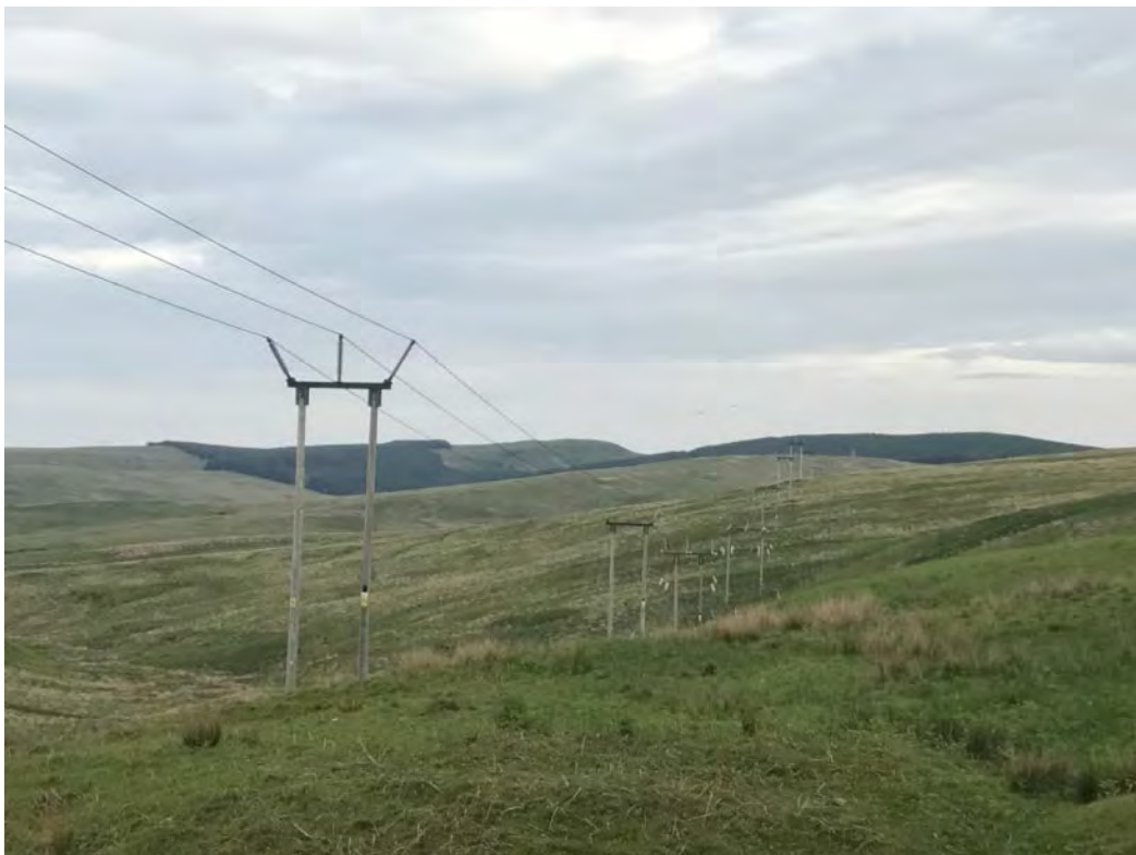
Figure 1.2: Example of a typical 132 kV H-pole trident OHL (SPEN, 2021)
