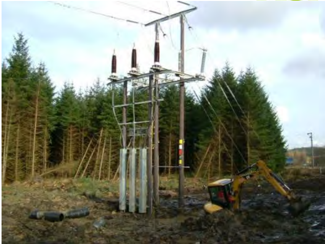
Figure 1.3: Example of typical terminal structures of a trident 132 kV OHL (SPEN, 2019)
