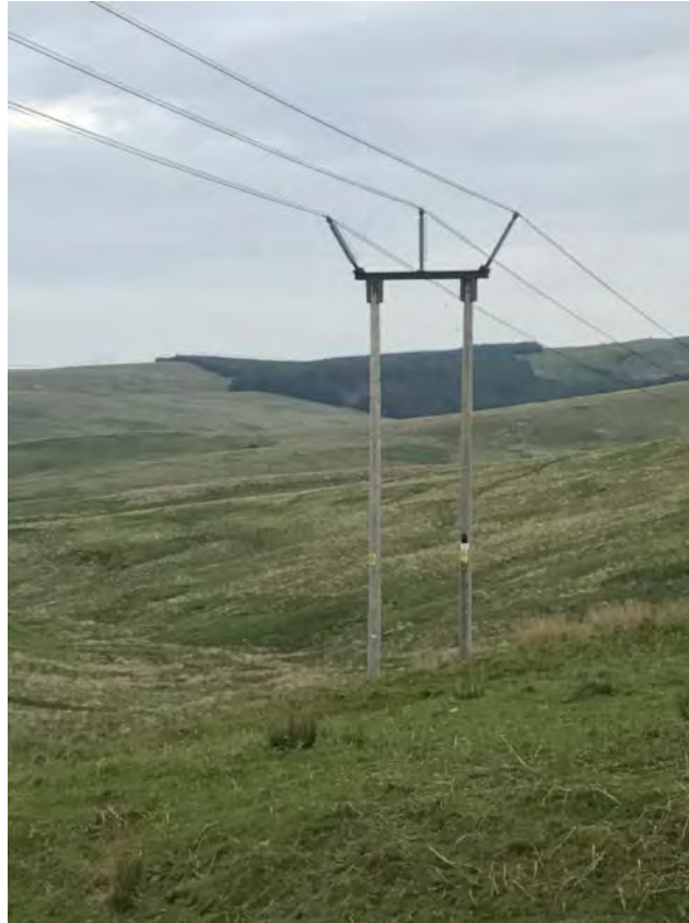
Figure 1.1: Example of a typical intermediate section of a trident wood pole supporting a 132 kV OHL (SPEN, 2021)
